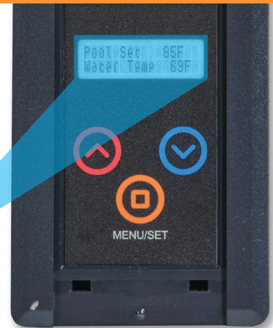
Control Panel Detail
